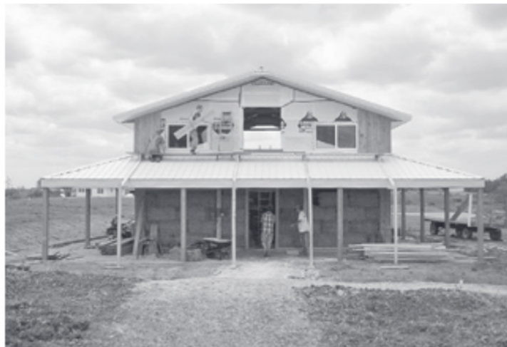
With the help of volunteers, the Sustainable Living Coalition in Fairfield, Iowa, built this straw-bale and post-and-beam barn for use as a classroom. (Submitted)
